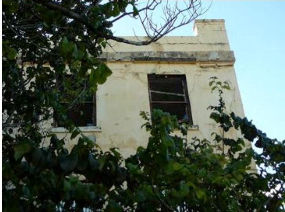
Figure 7. On the Nelson Place frontage there are signs of vandalism to windows but the main structure of the external wall appears to be in reasonable condition.
