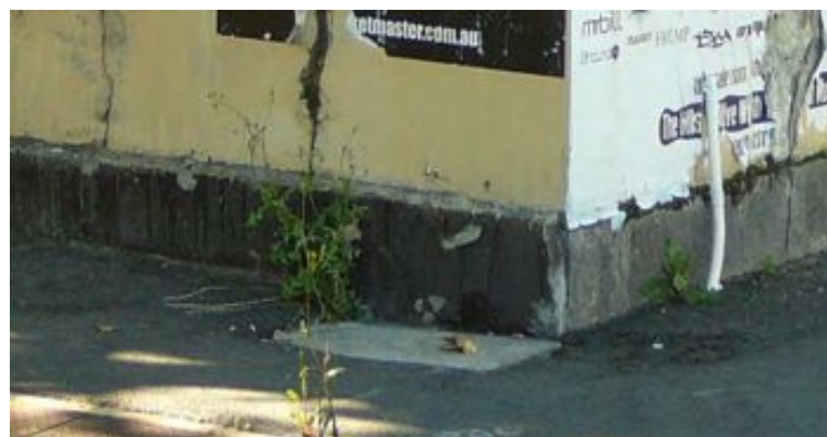
Figure 3. Large bluestone block foundations on corner of Nelson Place and Ann Street.
