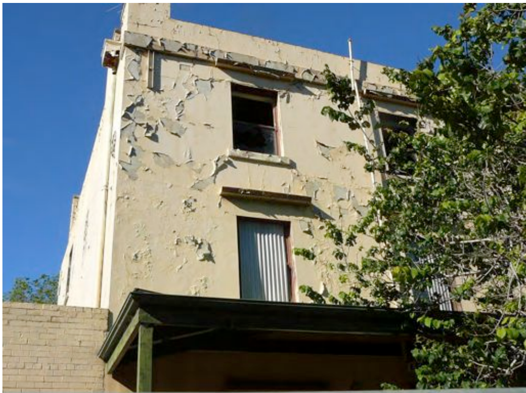
Figure 8. On the Nelson Place frontage the cement render is in good condition although the paint is peeling.
