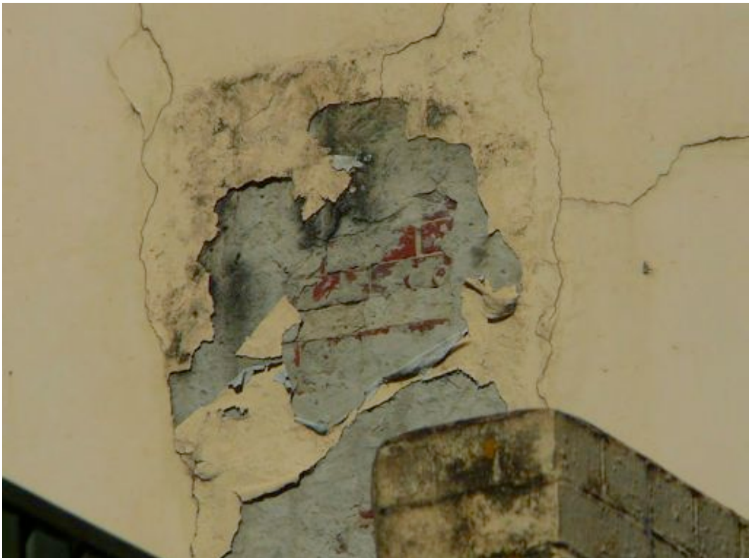
Figure 10. On the south-east side where a small section of render has fallen it is easy to see the brick construction on the south wall. The bricks are in good condition and the mortar joints are good.
