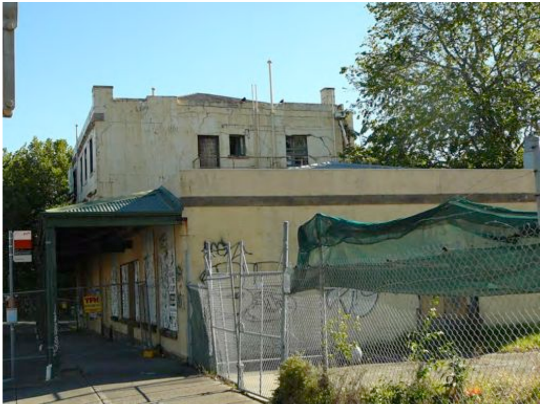
Figure 9. View of the south-west side, the rear of the Oriental Hotel. The verandah and ground floor addition in the foreground are not original.
